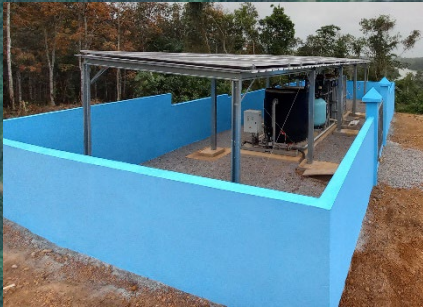
Treatment unit with photovoltaic roof and pumping to reservoir
