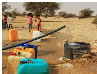
Mauritania – Flow rate tests on existing boreholes
