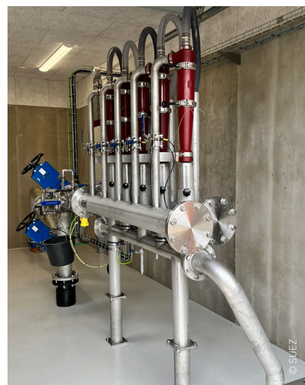
inDENSE implemented in Søholt WWTP (Denmark) in 2024.
