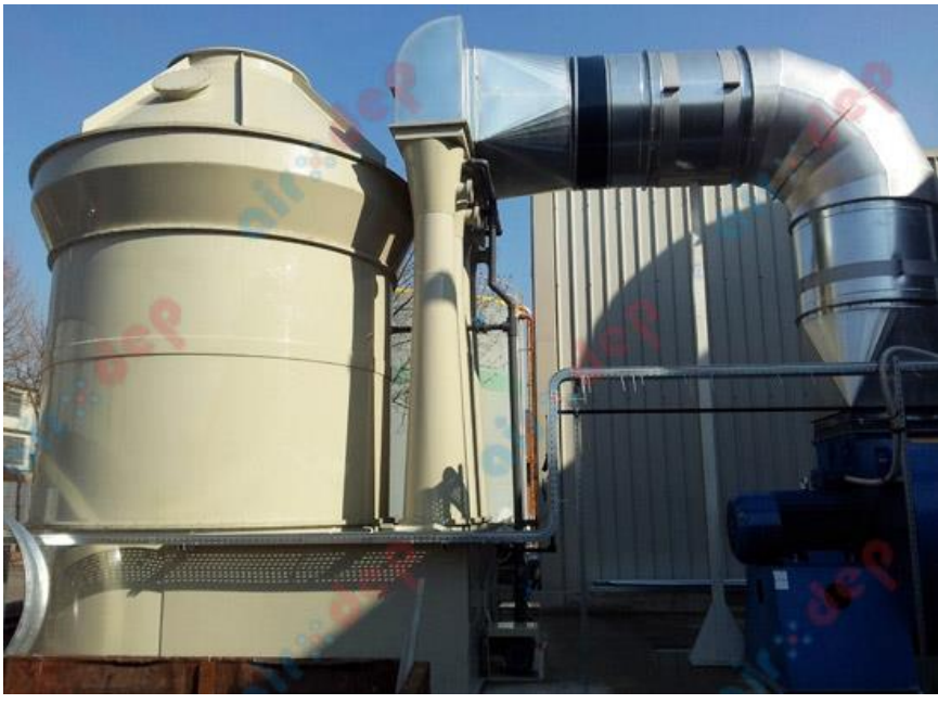
Scrubber venturi – SUEZ/AIRDEP
