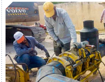
Infrastructures are severely damaged
