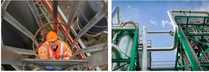
Solvent recycling and recovery facility in Almelo, Netherlands/ Credits: SUEZ
